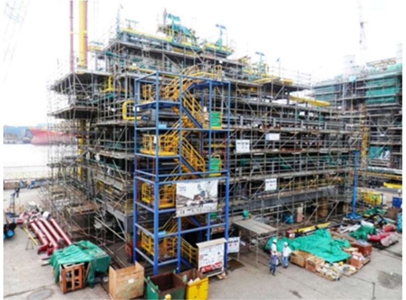
HP/LP Separation Module
